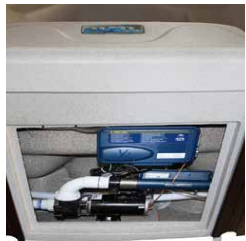
Equipment access is below the topside control panel on most spas.
