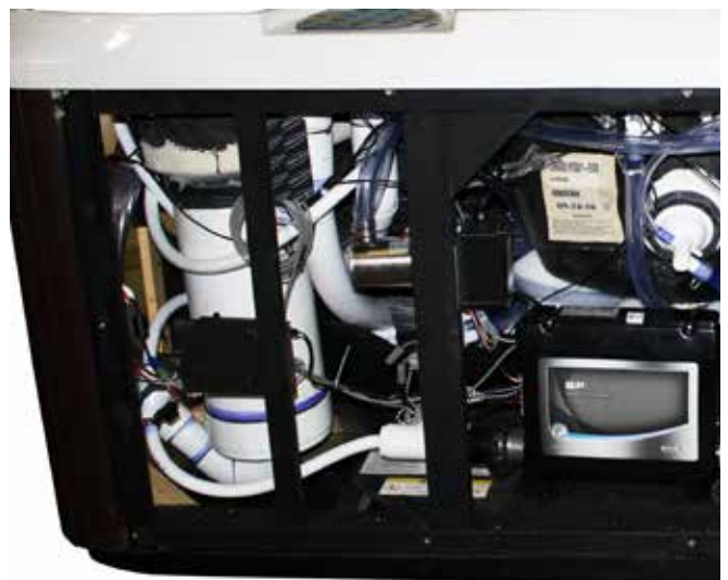
Equipment access is below the topside control panel.
